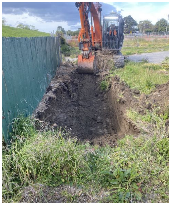
Diggers were used to remove all traces of alligator weed from the Marsden Street site.
